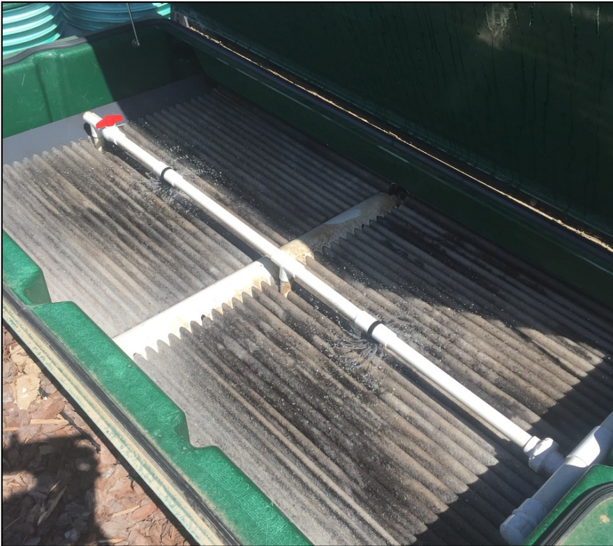
Spinner Nozzles Check spray coverage
